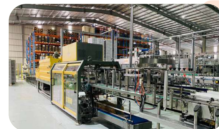
Ceylon Beverages Total Electrical Services
